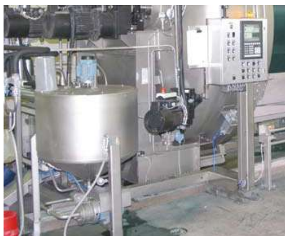
Preparation tank & main panel
