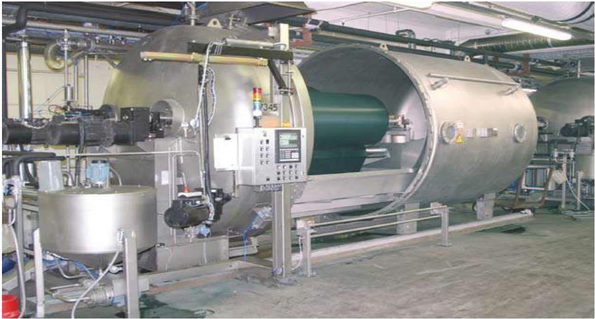
Modernized High Temperature Jigger machine
