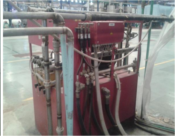
Open Thermic oil and steam valve
