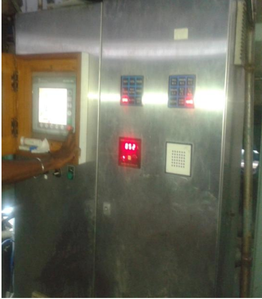
Operating Main panel
