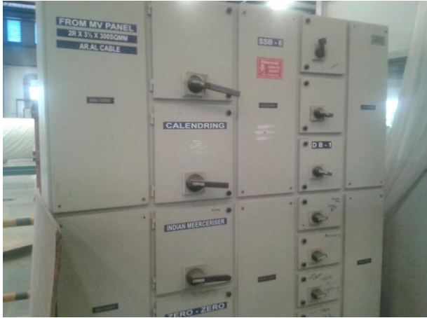
Switching on the Power
