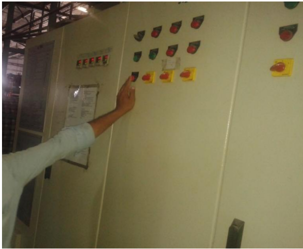
Switch ON the main on panel
