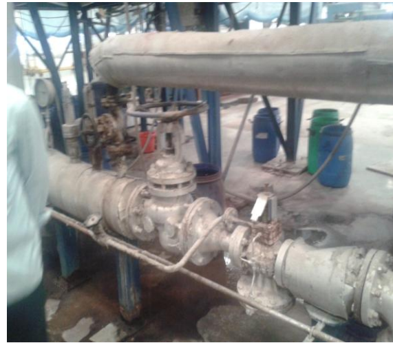
Open the steam, water and air valve
