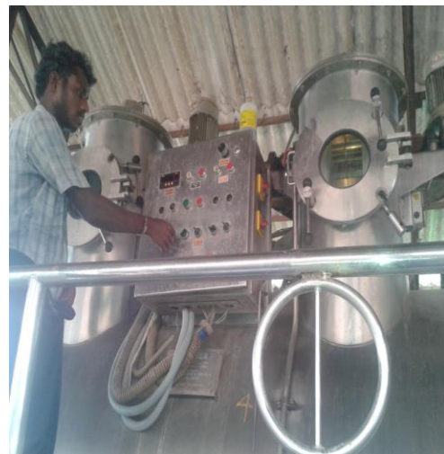
Operating main panel
