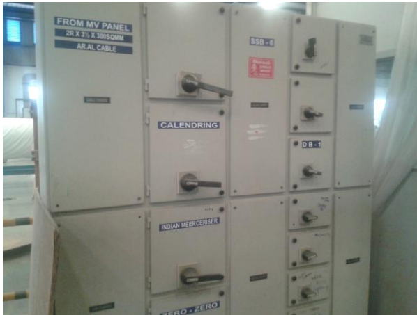
Switch ON the Main power
