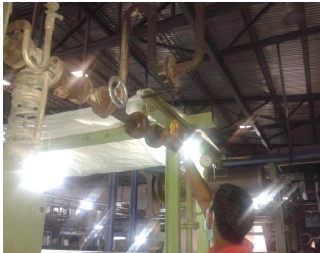
Opening of steam valve
