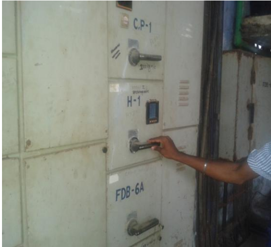
Switching ON main panel
